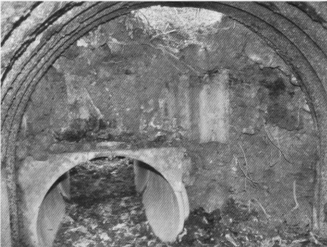
Inside Ashburnham OP with emergency exit, viewing point and remaining section of corrugated-iron end wall
